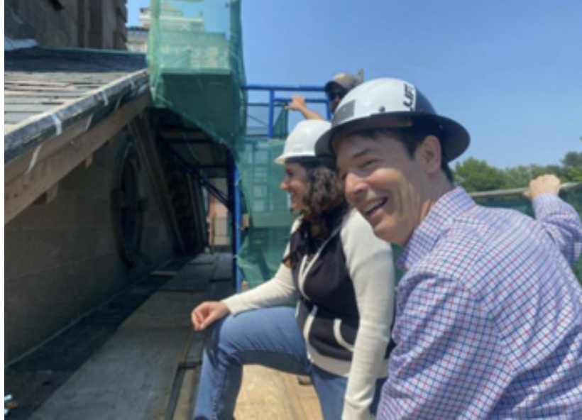
Restoration Committee Chair Jon Andersen-Miller, perched on the scaffolding high above Arlington Street, approving paint colors ... and pretending his legs haven't turned to Jell-o!
