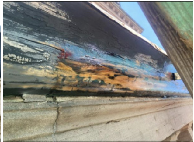
And then getting a coat of primer. They'll have a finish coat of "brownstone" brown to blend back in, possibly with stone dust mixed in for texture.
