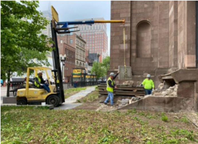
Stone being removed and taken to the mason's stone yard for recycling as "dutchmen" for front facade and stairs
