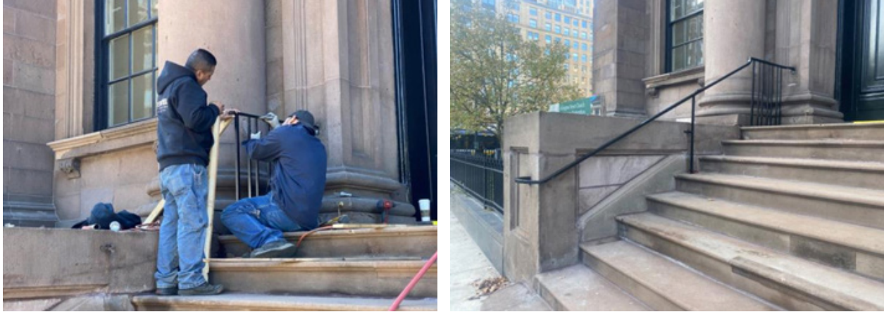
This week our restored iron handrails returned! Also note the restored brownstone behind them! All thanks to Restoration Committee Chair, Jon Andersen-Miller
